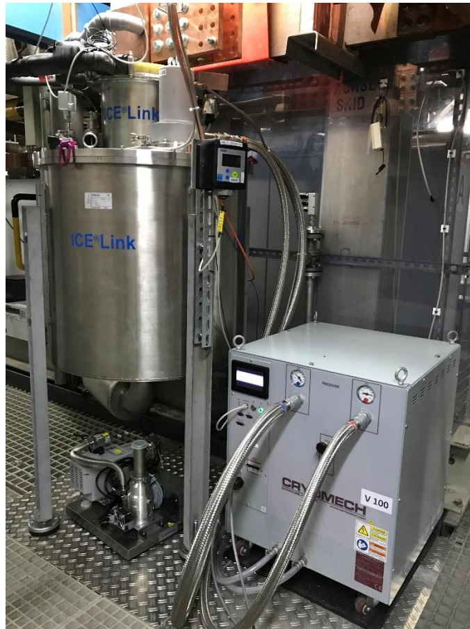
Figure 9 20 kA current lead used in the 3S project. Left: current lead with copper connections at the top, HTS connection at the bottom. Right: compressor used for cryocooler.
