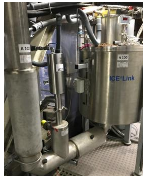
Figure 4: Current lead with connected superconducting busbar
